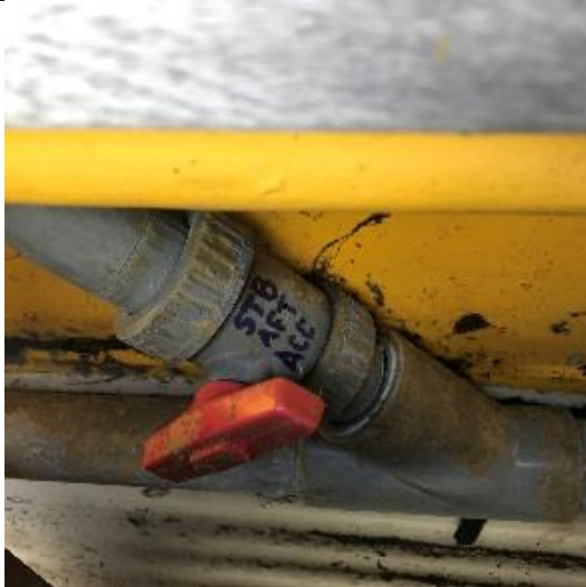
Aft accommodation valve
