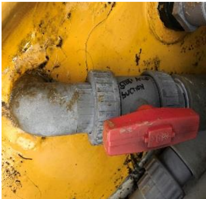
Forward accommodation valve
