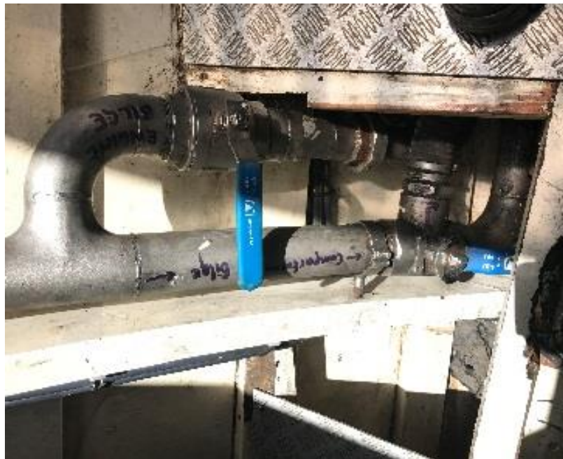
Engine room valve
